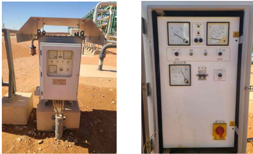
Fig. 2. Cathodic protection system cabinet after its opening and current stimulation from control room
